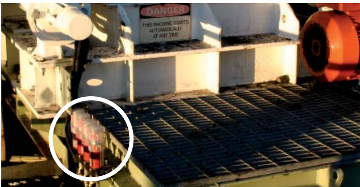
Lubrication of various bearings on a coal crusher. perma STAR made it possible to install the lubrication point outside the danger zone.
