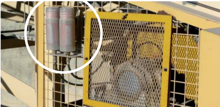
The remote installation of perma STAR VARIO lubricators to this conveyor pulley bearing at a cement plant has allowed the hole in the guarding to be repaired. The lubricators can be inspected and serviced safely while equipment is running which has improved safe work practices and saved time.
