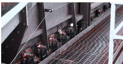
Bearing lubrication at tree sorting system
