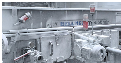
Bearing lubrication of a belt thickener
