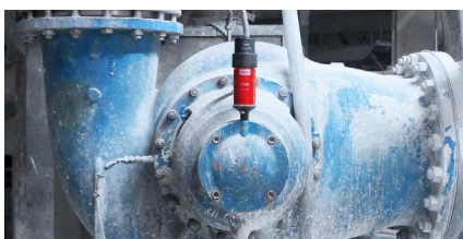
Bearing lubrication on a pump
